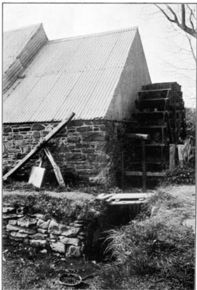
Fig. 5. The Llanrhystyd Yarn Factory. The undershot waterwheel and sluice-gate. Note the floodgate lever (which is manipulated from inside) projecting from the gable end of the building.
