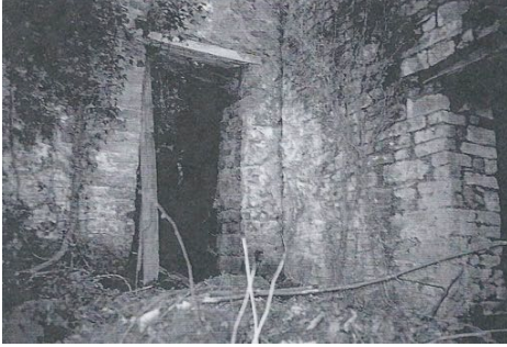
PLATE 21 The join between the two walls is evidence that the kiln building (on the right) was a later extension
