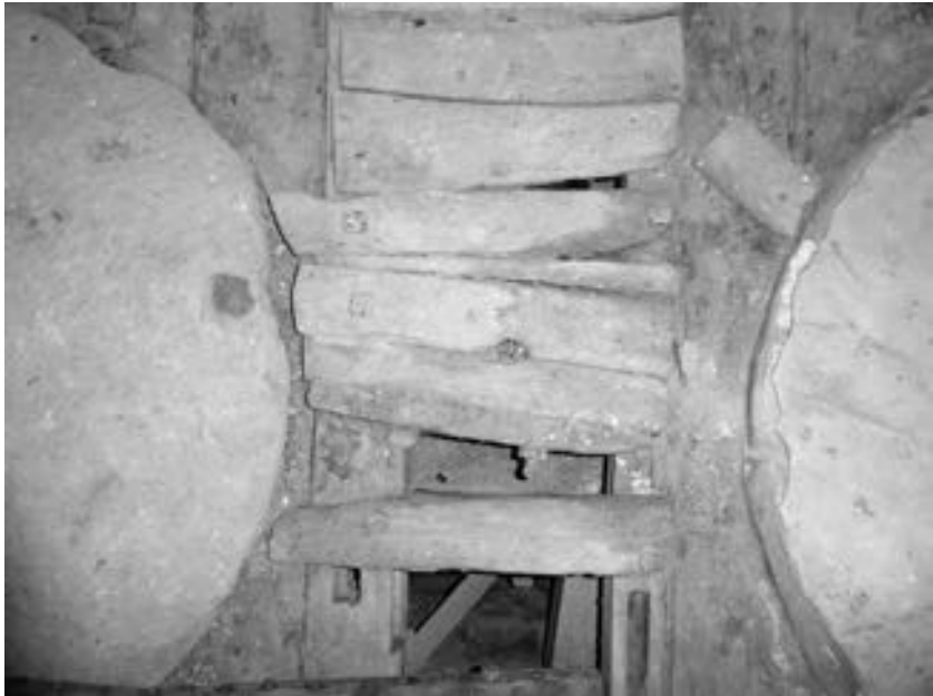
PLATE 6 The timbering supporting the top of the upright shaft, from above. The bedstone is on the right-hand side
