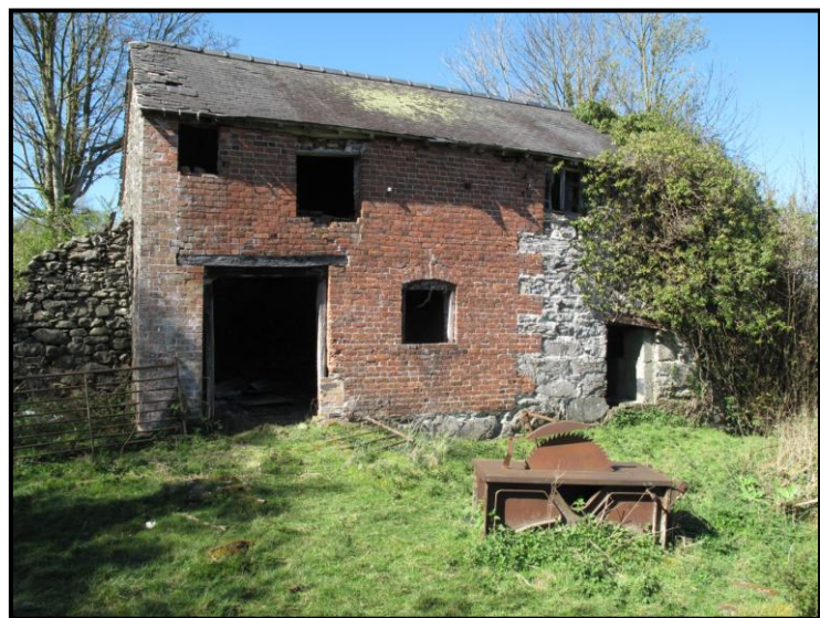
Melin-y-grug showing the extensive brick repairs to the front wall
